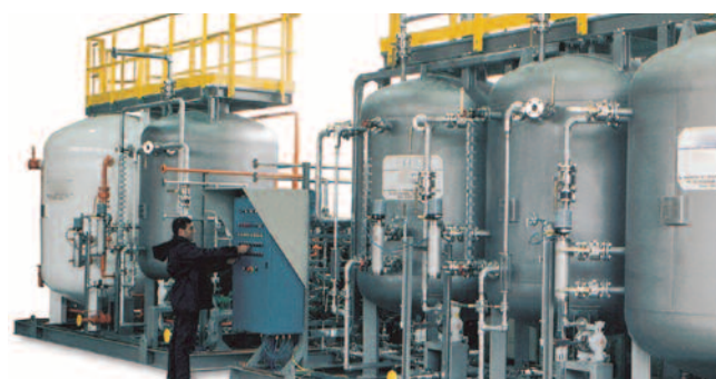
Sulphuric Acid, Biodispersant, Scale Inhibitor and Biocide Dosing Package.
