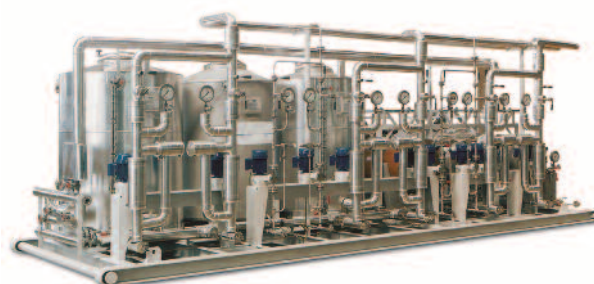
Chemical Dosing Package.
